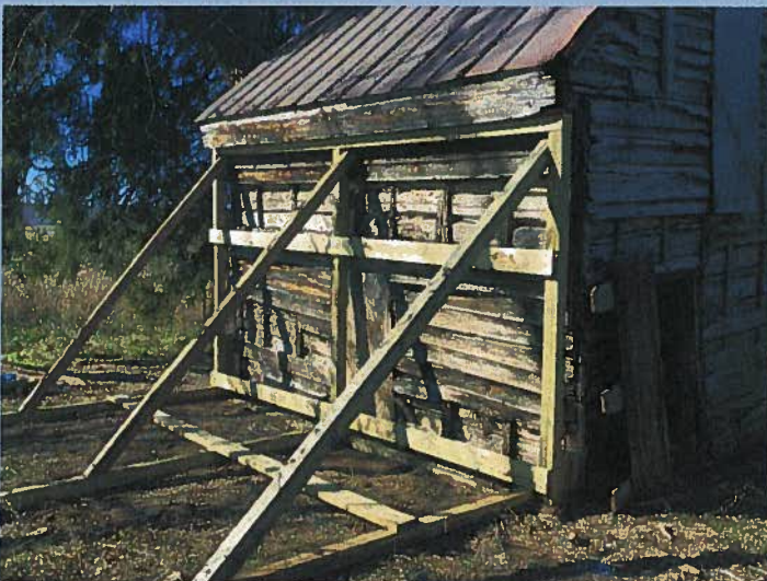
Work has been done to shore up the slave quarters as well as to protect from termites.
